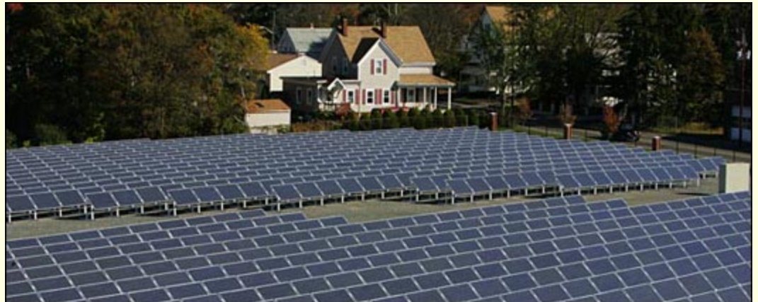
Solar panels at Brockton, Ma. Brownfields site
